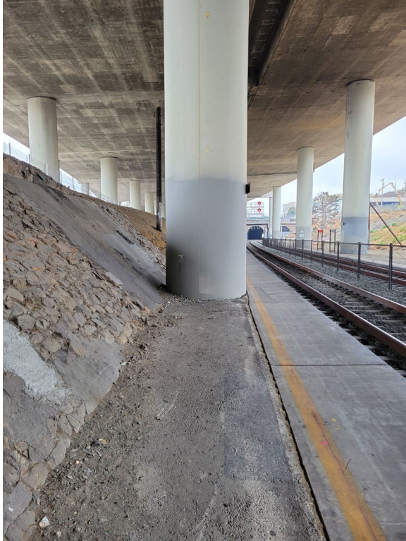
Figure 4 Northbound Platform Circulation: I-280 Column Obstruction
