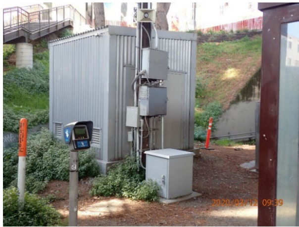
Figure 11 Southbound Sump Pump House
