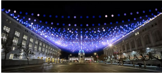
CIVIC CENTER/UN PLAZA CATENARY LIGHTING
