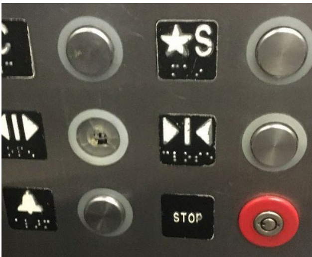
Figure 8. Vandalism to destination buttons at Powell St. Station platform elevator, December 2021.
