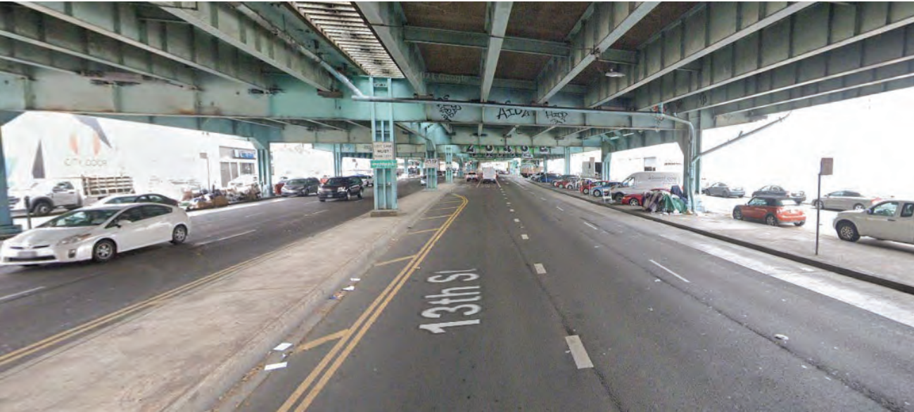
13 th Street between South Van Ness Avenue and Folsom Street, facing west
