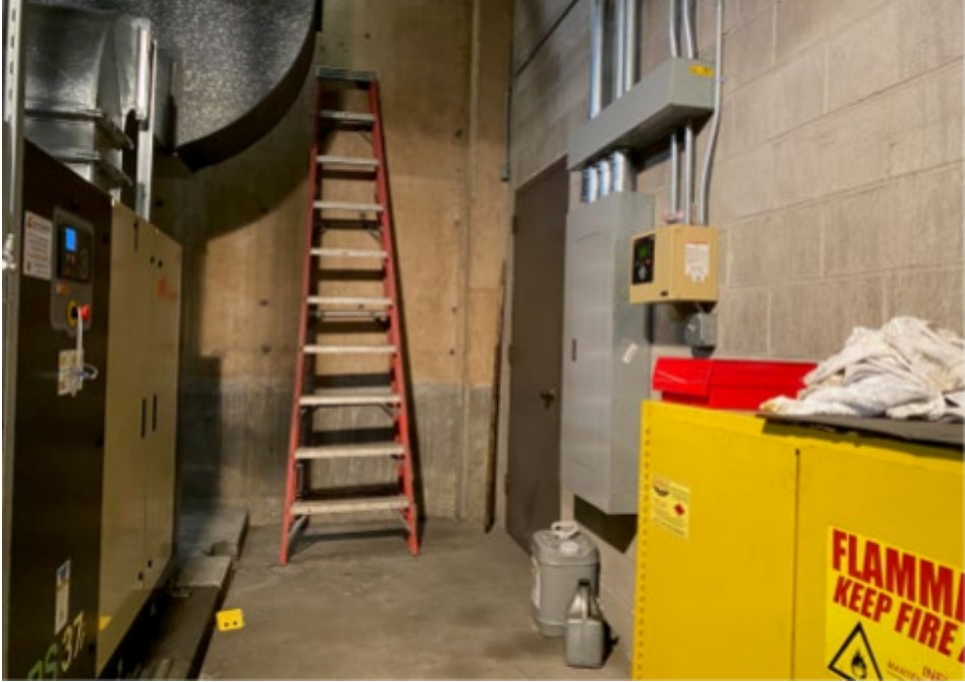
Photo 10: Existing Green Car Wash Electrical Power Room (at the basement)
