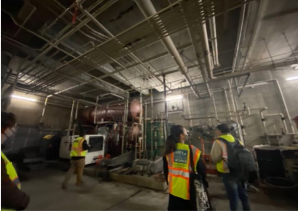
Photo 8: Existing Green Car Wash Machine and Pump Room (at the basement)
