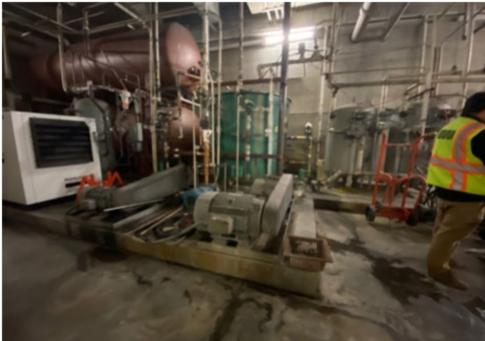
Photo 2: Existing Green Car Wash Machine and Pump Room (at the basement)
