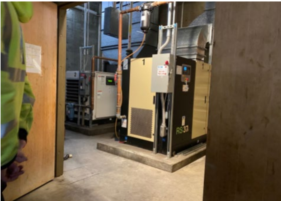
Photo 9: Existing Green Car Wash Electrical Power Room (at the basement)
