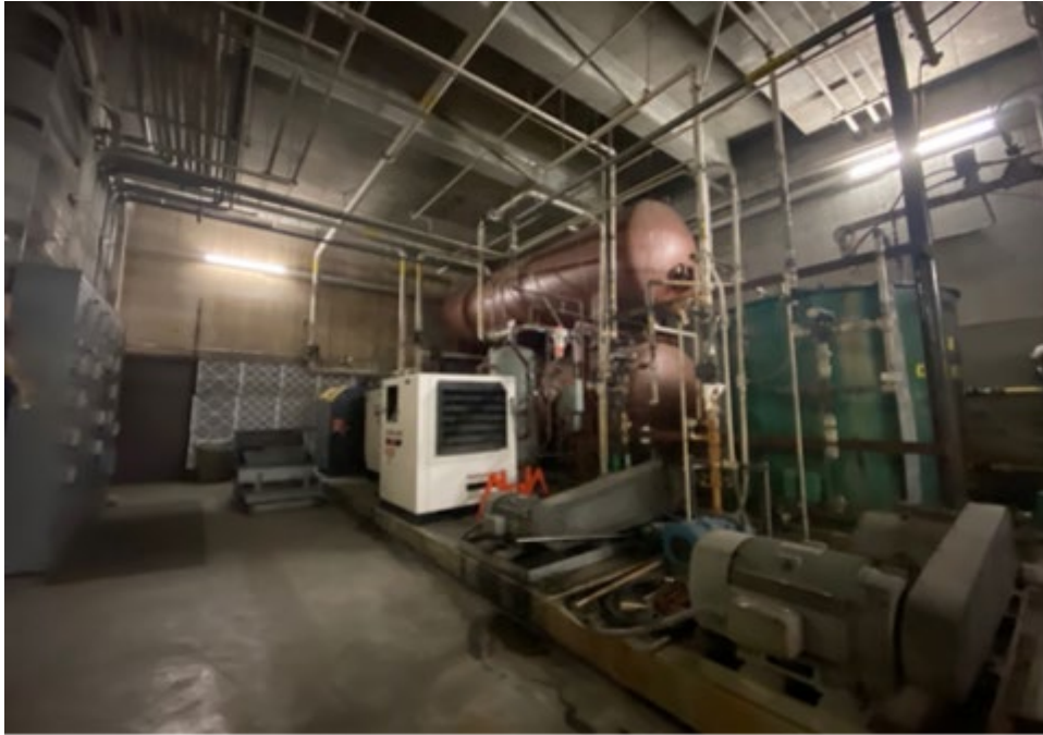
Photo 1: Existing Green Car Wash Machine and Pump Room (at the basement)
