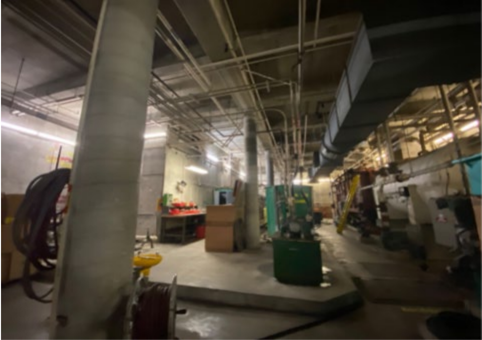
Photo 6: Existing Green Car Wash Machine and Pump Room (at the basement)
