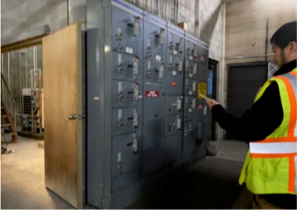
Photo 11: Existing Green Car Wash Electrical Power Room (at the basement)
