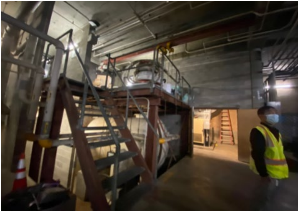
Photo 5: Existing Green Car Wash Machine and Pump Room (at the basement)
