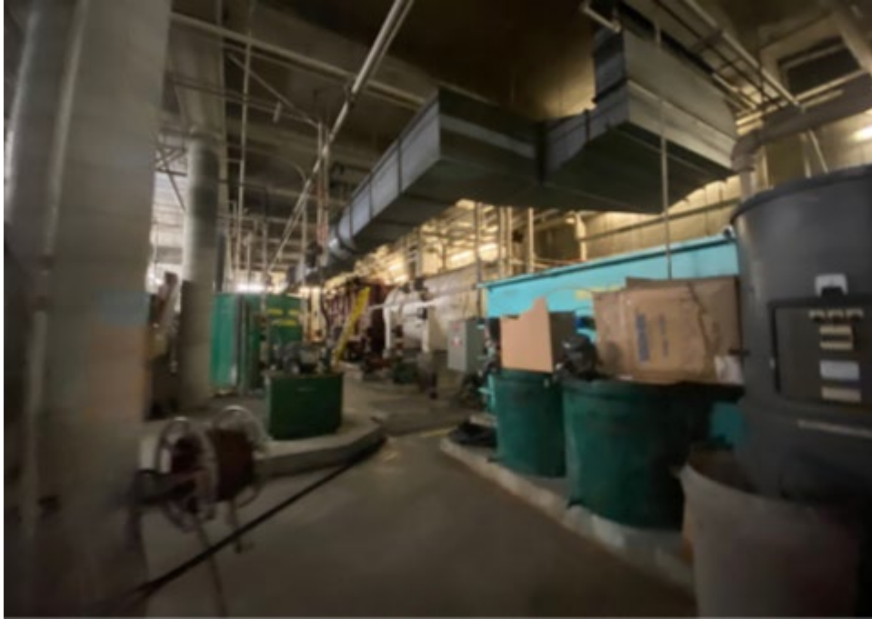
Photo 3: Existing Green Car Wash Machine and Pump Room (at the basement)
