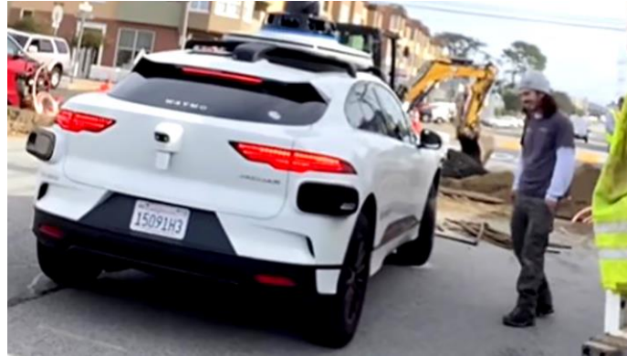
Intrusions into work zones endangering workers
