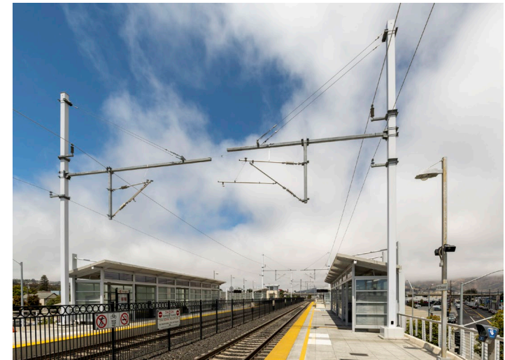
Overhead Catenary System
