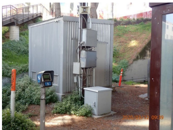
Figure 11 Southbound Sump Pump House
