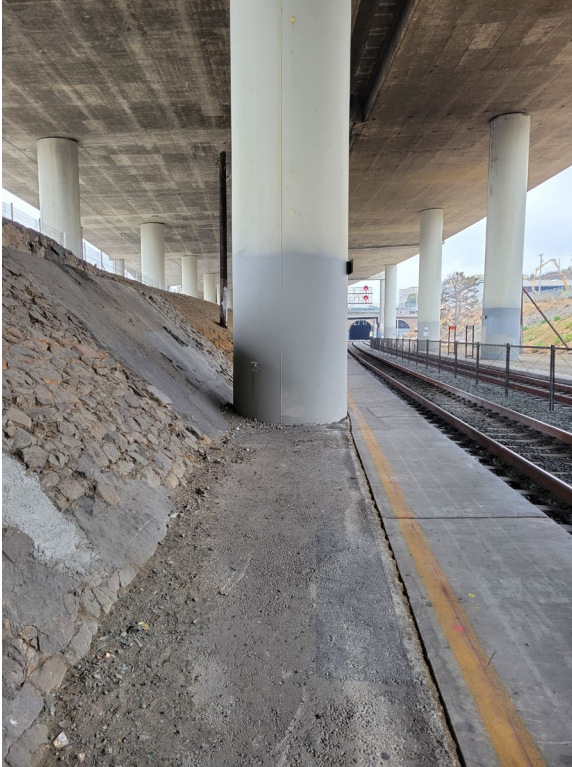
Figure 4 Northbound Platform Circulation: I-280 Column Obstruction
