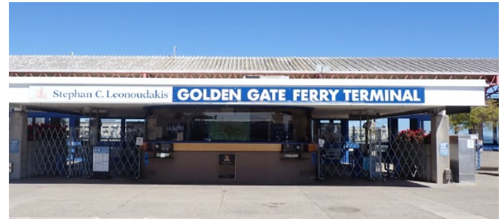
Current Port fencing condition: South building
