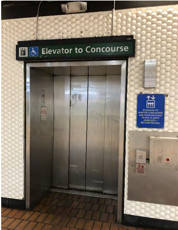
Figure 7. Door vandalism and deterioration of platform elevator at Powell St. station, December 2021.
