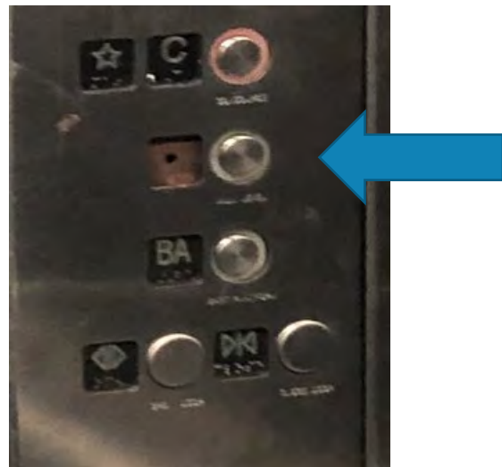
Figure 6. Vandalism to destination buttons at Civic Center Station street elevator, December 2021.
