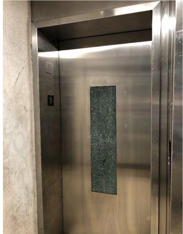
Figure 8. Shattered window glass of platform elevator at Civic Center station, December 2021.
