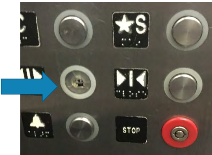
Figure 5. Vandalism to destination buttons at Powell St. station platform elevator, December 2021.
