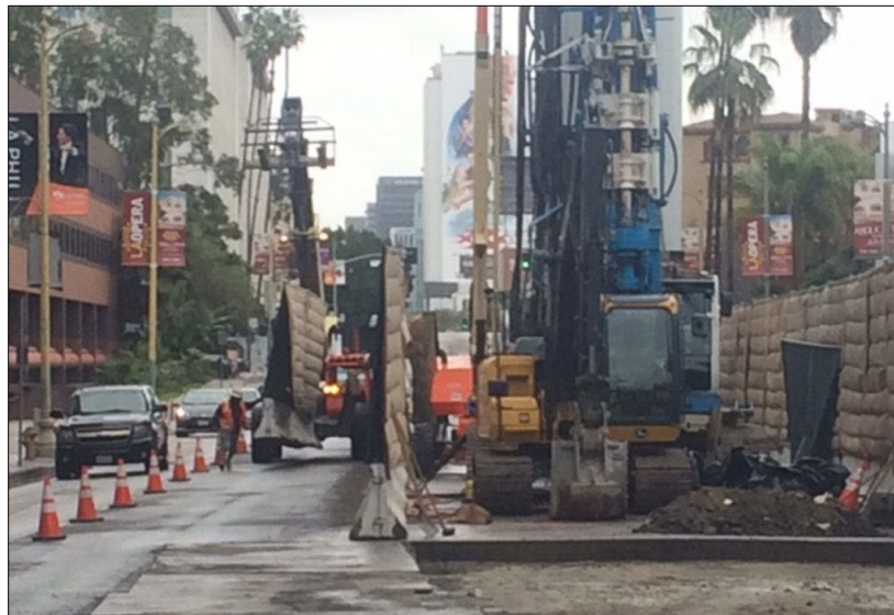
Figure 7-16. Example of Footprint Required for Jet Grout Operations from Surface and Associated Traffic Control (LA Metro Purple Line)
