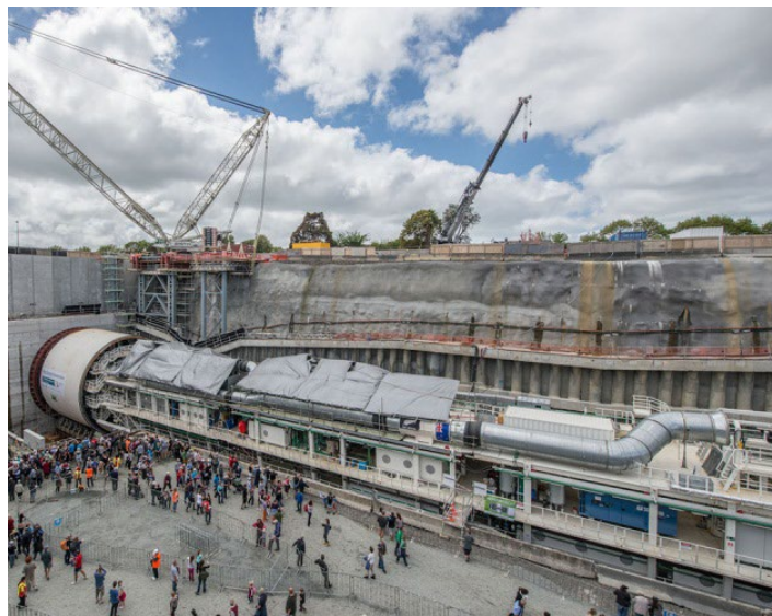
Figure 7-7. Example of a TBM Set Up and Ready to Excavate into a Headwall (46-foot-diameter TBM, Waterview, NZ)
