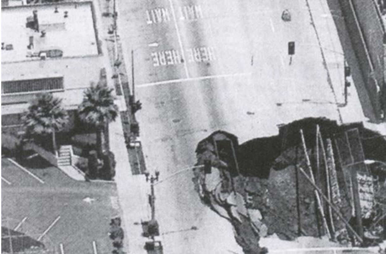
Figure 2: Traffic Decking for the Red Line at Hollywood Blvd./Highland Ave. in Los Angeles
