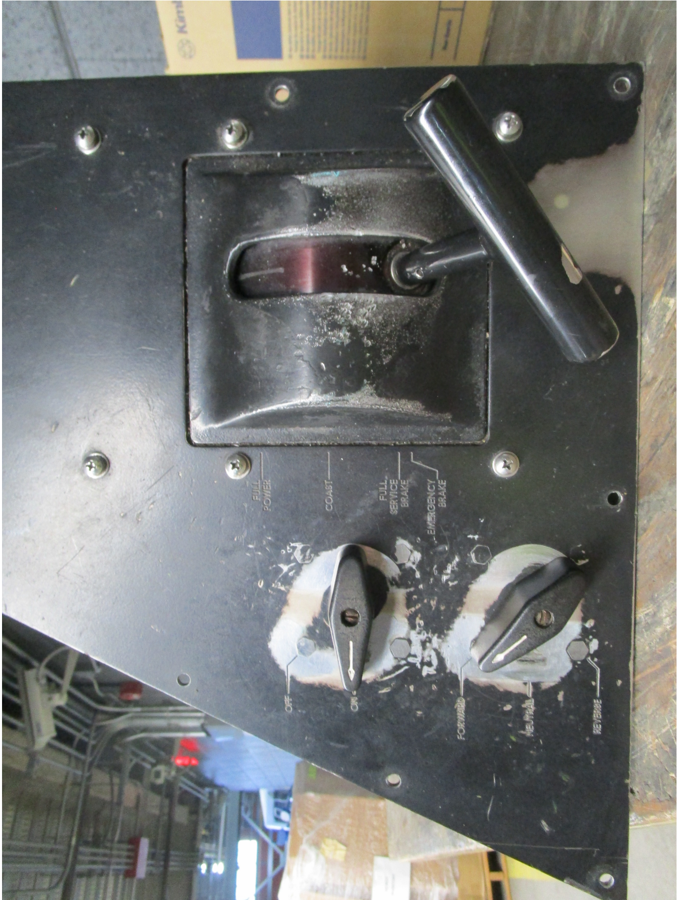
Breda LRV Master Controller - Existing Condition
