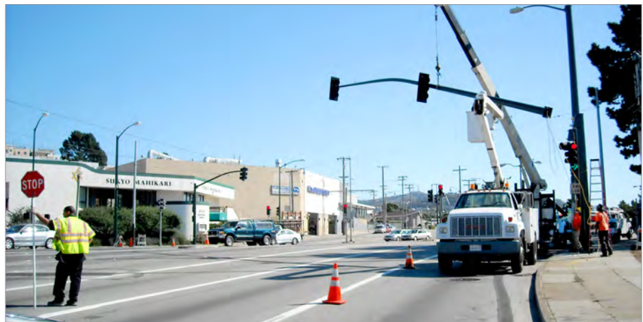
New signal installation is part of the 19th Avenue Combined City Project. ▲
