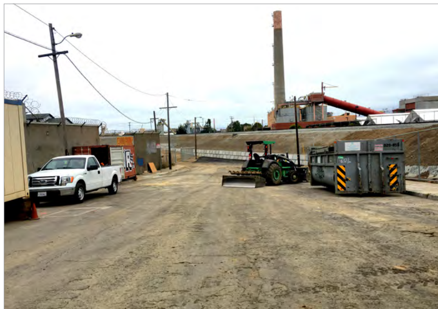
The earthen berm replacing the old Quint Street Bridge is in place and connector road construction could begin in 2018, pending final acquisition of the land. ▲
