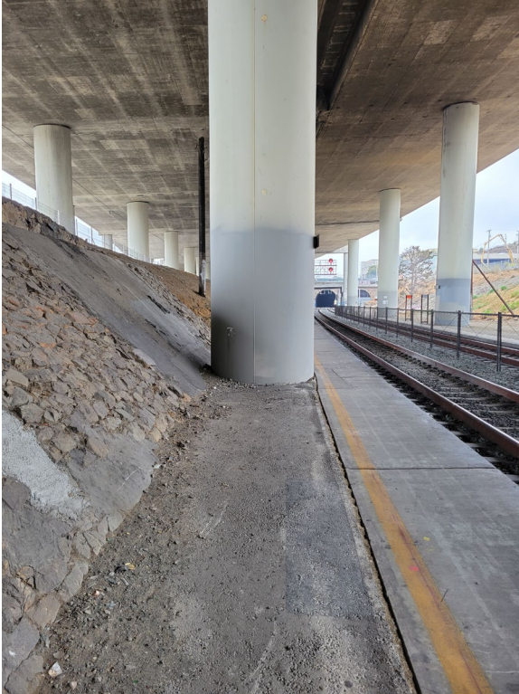
Figure 4 Northbound Platform Circulation: I-280 Column Obstruction
