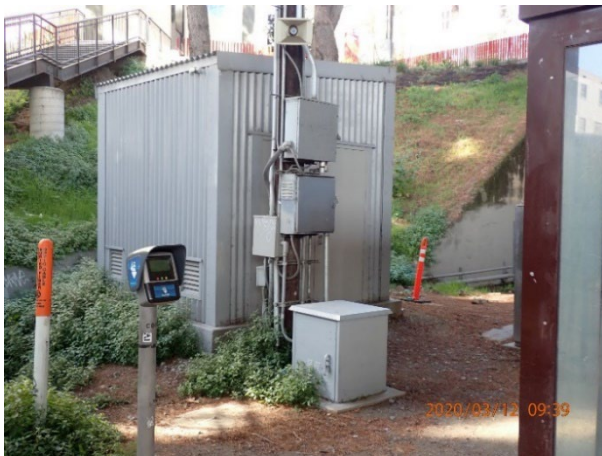
Figure 11 Southbound Sump Pump House
