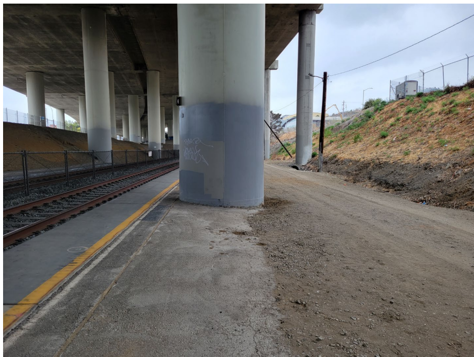
Figure 13 Southbound Platform Circulation Obstruction by I-280 Column
