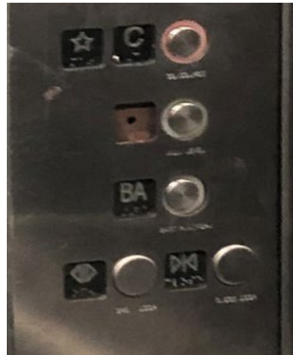
Figure 9. Vandalism to destination buttons at Civic Center Station street elevator, December 2021.
