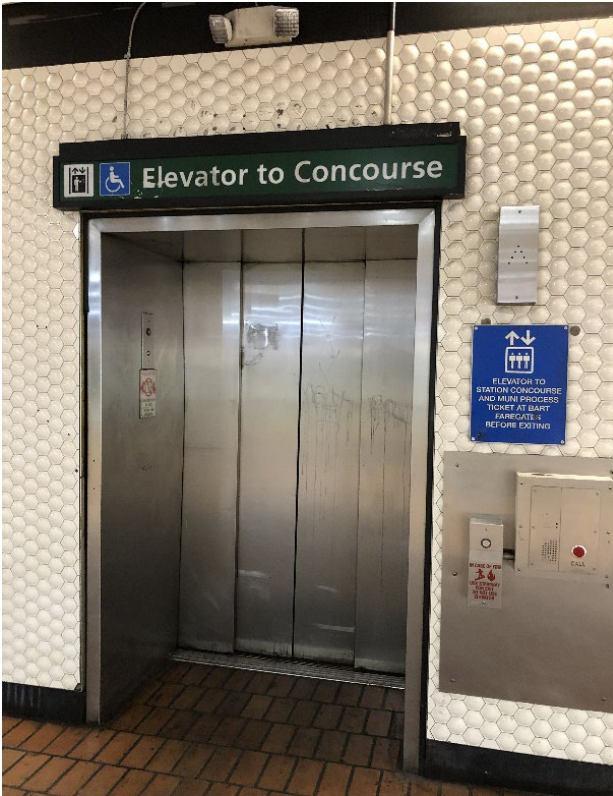
Figure 9. Door vandalism and deterioration of platform elevator at Powell St. Station, December 2021.
