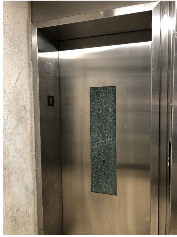
Figure 10. Shattered window glass of platform elevator at Civic Center Station, December 2021.
